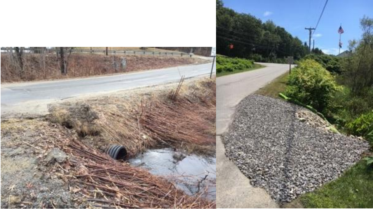
Figure 6. Unstable stream culvert at south end of site, before and after.
