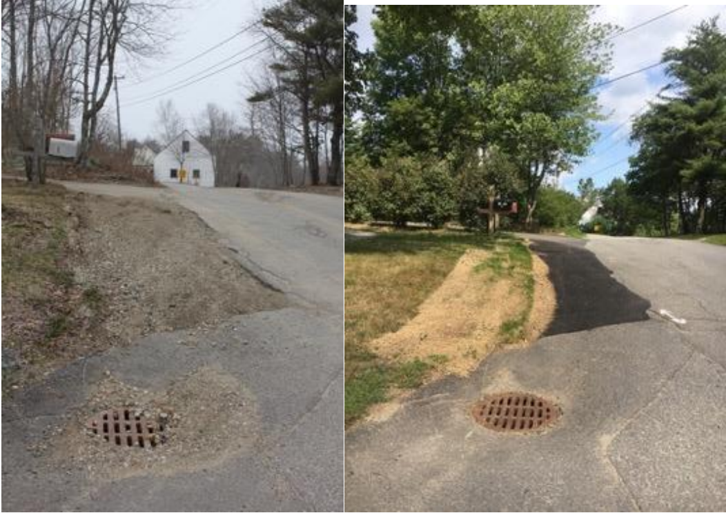
Figure 5. Eroded road shoulder at north end of road was paved and stabilized and seeded.
